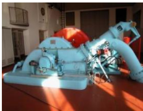
Photo 2. Mühlau: Drinking water turbine (2-nozzle Pelton turbine).
