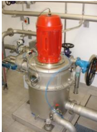
Photo 33. Counter pressure Pelton turbine (Fällanden SHP plant, Switzerland, set in a drinking water network, H = 140 m, Q = 16 l/s, P = 17 kW, 2008).
