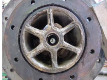
Photo 30. The x-cross liner for a nozzle, worn out by limestone.
