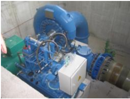
Photo 25. Francis turbine with a spiral casing (case study Sangüesa).
