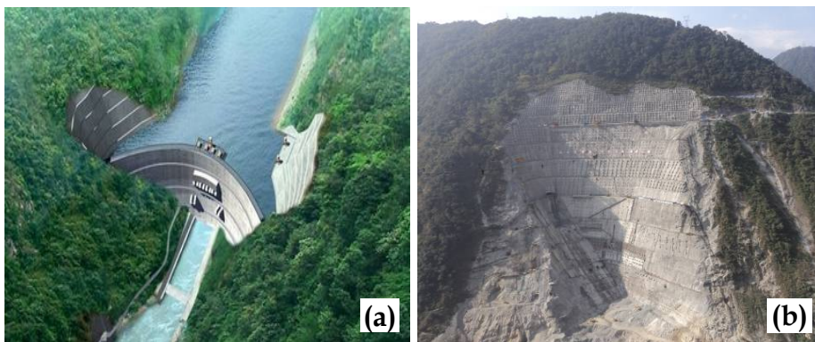
Fig. 12. Geomorphic photograph of the dam site: (a) The layout of key water control, and (b) The right bank slope after excavation.
