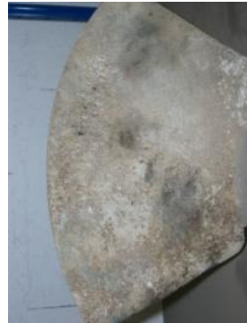
Photo 36. A Kaplan turbine blade, manufactured without hydraulic laboratory techniques, eroded by cavitation after a few months operation.
