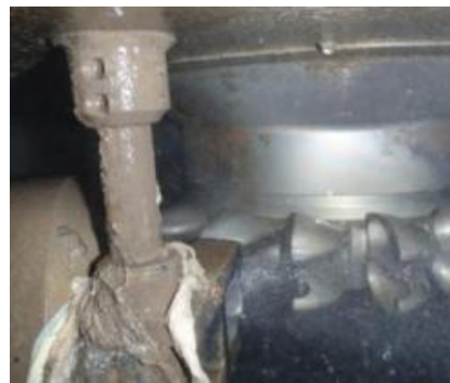
Photo 38. A deflector in the raw wastewater (case study le Châble Profray).
