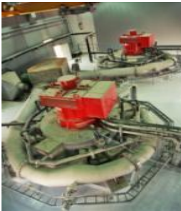
Photo 13. Two 5 nozzle Pelton turbines set on the raw wastewaters of Amman City, As Samra plants (Jordan) ( H = 104 m, Q = 2 \times 1.25 m 3 /s, P = 2 \times 830 kW, E = 12.5 GWh/year, 2007).
