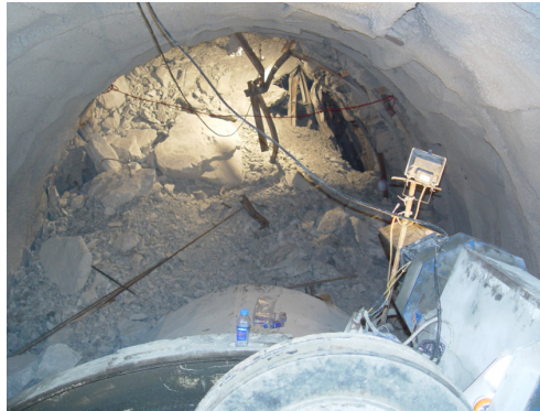
Fig. 21. The damage phenomenon of tunnel and TBM after rockburst on November 28, 2009.
